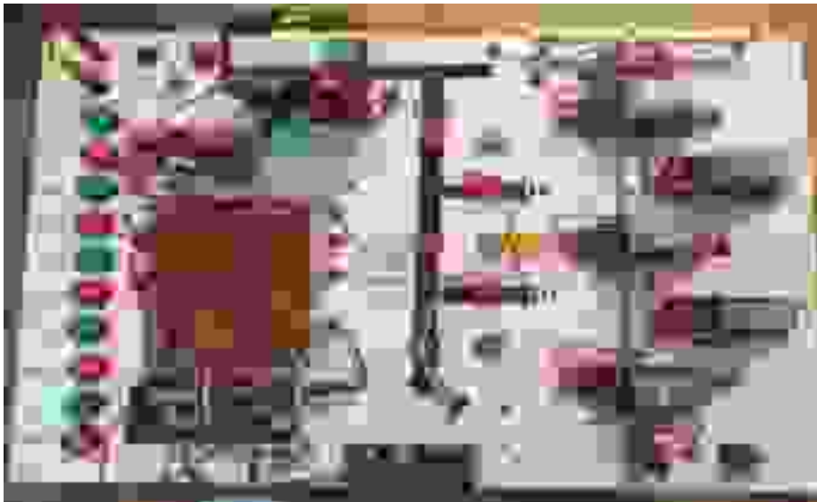
Fig: 6 220kv feeder management unit
